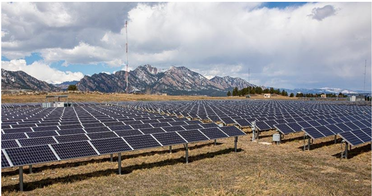
The 1-MW photovoltaic array at NREL's Flatirons Campus. Photo by Werner Slocum, NREL
